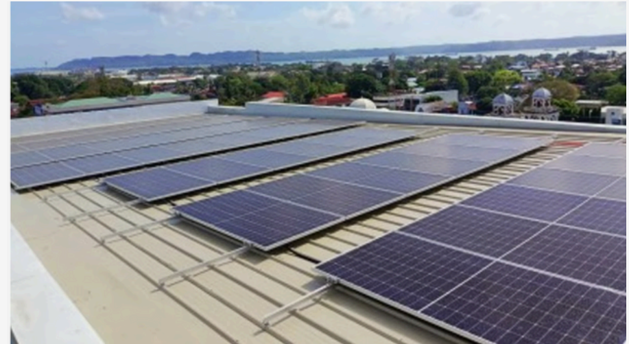
SOLAR POWER. Iloilo City Hall adopts solar energy. The power generated by the 134 solar panels is expected to generate 60 kilowatts a day and will provide around one-third of the power demand at the city hall. PNA PHOTO
